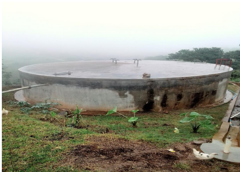
Photo 2: A water tank and stand pipe on Sankhulani GFS in TA Nsabwe (Useful technology in hilly and dry areas)
